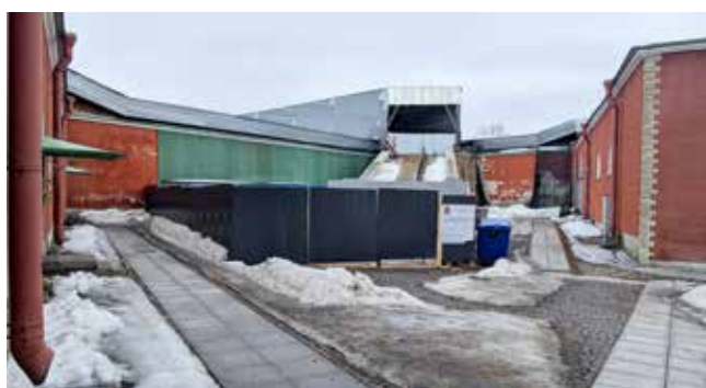
Fig. 6: The Menshikov Bastion of the Peter and Paul Fortress under construction for the Museum of the History of St. Petersburg, February 25, 2024. Photo: Authors
