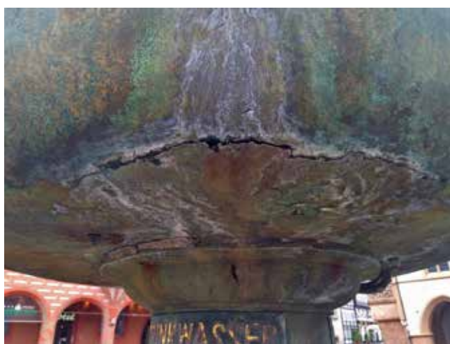
Fig. 9: The crack in the upper bowl of the market fountain.
