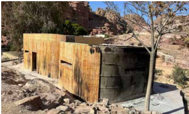
Fig. 2: Burned visitor’s facilities. Photo: Sela for Training and Protection of Heritage
