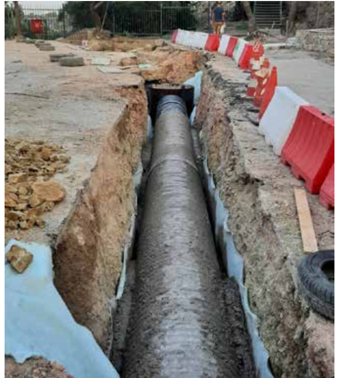
Fig. 4: Big plastic pipe buried to the south of the Areopagus, part of the drainage network. View of the ditch looking west. The big pipe is being encased in cement that will bear the fill to reach the surrounding ground level. (March 2023)
