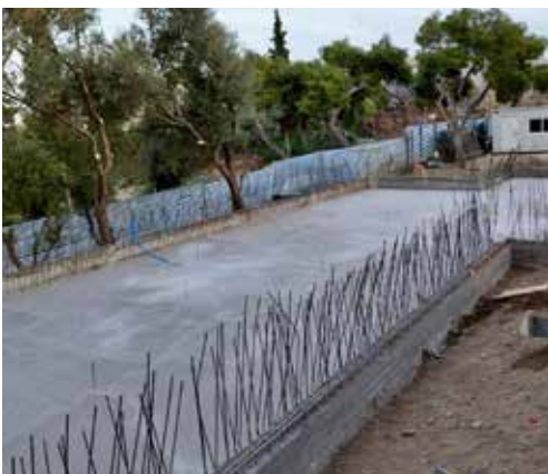
Fig. 7: A closer view of the foundations of the new ticket office from the southeast. Above on the right, the rock of the Areopagus. (2024)
