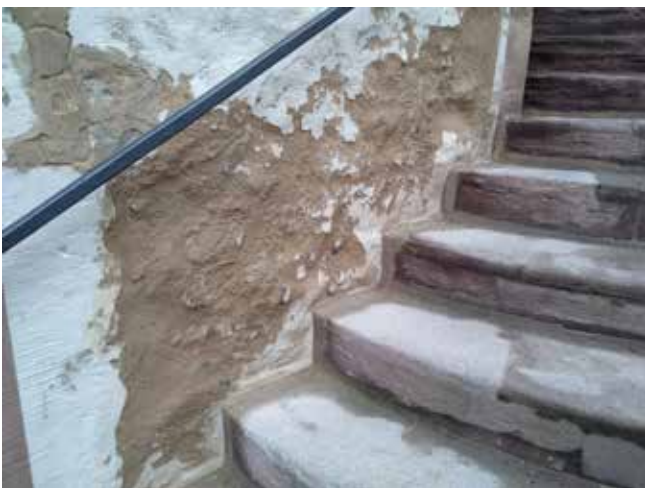
Fig. 4: The outside wall of the City Hall exhibits serious humidity after a 12-year restoration which had cost 14.4m EUR. Photo: Henning Frase
