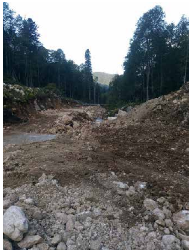
Fig. 6: Destruction caused by the construction of a water pipeline. Photo: The authors
