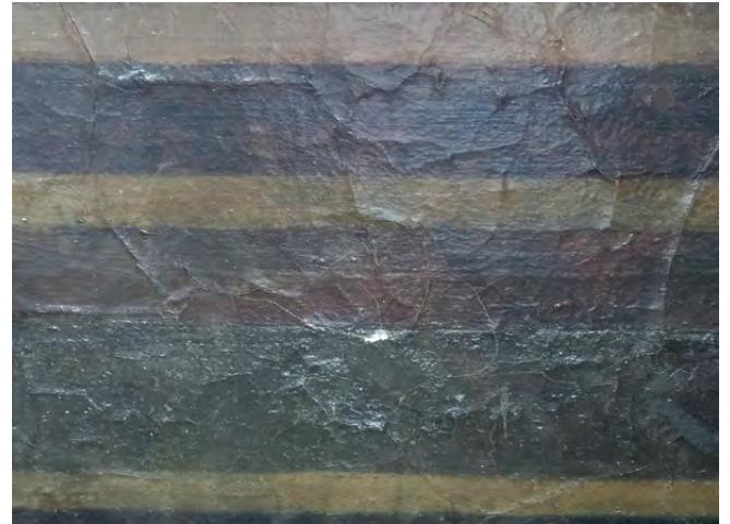
Fig. 5: The wall paintings of the Emperor's Hall, the main room of the Imperial Palatinate, show extensive flaking. Photo: Henning Frase
