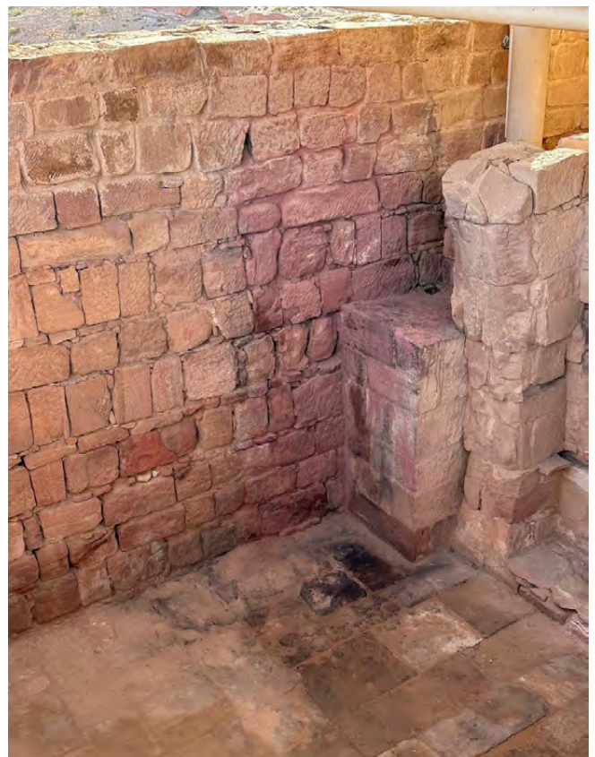
Fig. 4a, b: Fire residues at the Byzantine church after emergency intervention. Photo: Sela for Training and Protection of Heritage
