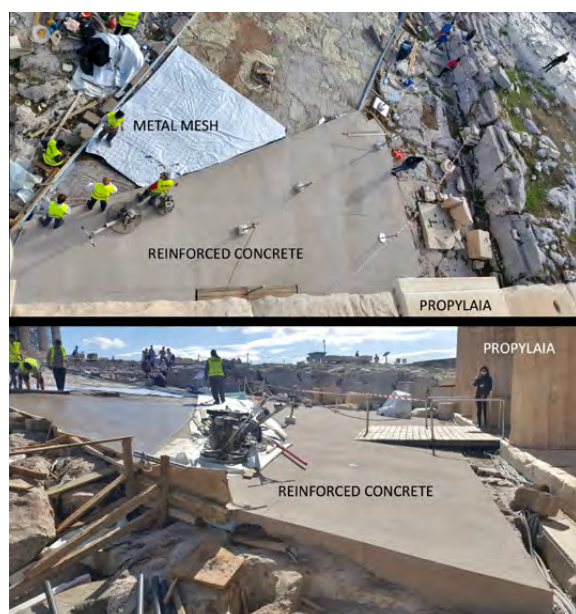
Fig. 1: Paving the rock to the east of the Propylaea. Above: The metal mesh spread on the white plastic sheet resting directly on the living rock. Below: To the right at the bottom of the picture, the thickness of the reinforced concrete resting on the living rock. (October 2020)
