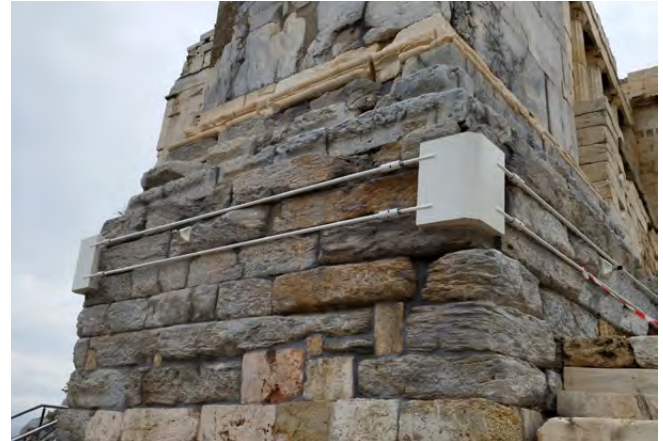
Fig. 11: “Consolidation” of the Agrippa Pedestal. Prestressed rods, framing the periphery of the course on top of the foundation. Two prestressed rods inserted in cylindrical holes that are straight through and enter and exit on the external surfaces of the course. (2023)
