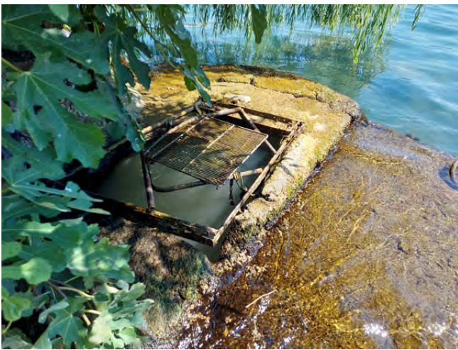
Fig. 5: Visibly defective sewerage infrastructure near the Saint Sophia church in Ohrid leaks into the world's most species rich lake in terms of endemic taxa to surface area. (Ohrid SOS, Aug. 16, 2023)
