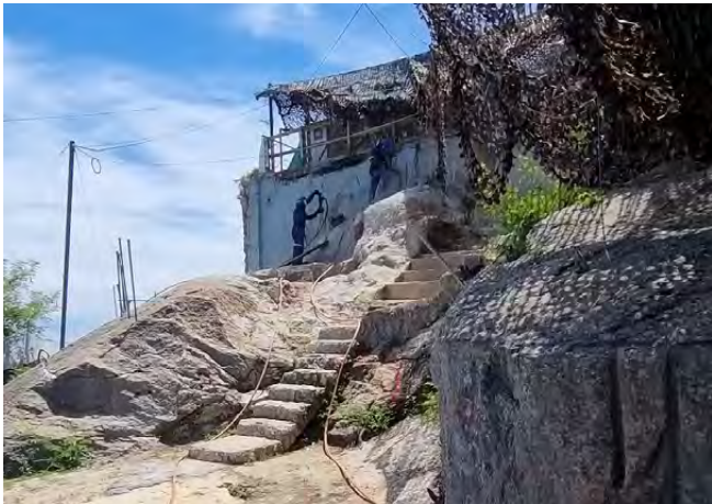
Fig. 3: The image which caused a stir in Rio de Janeiro when publicized: the removal of dozens of cubic meters of rock from the top of Sugar Loaf for the construction of the upper station of the zipline. Photo: Movimento Pão de Açúcar sem Tirolesa
