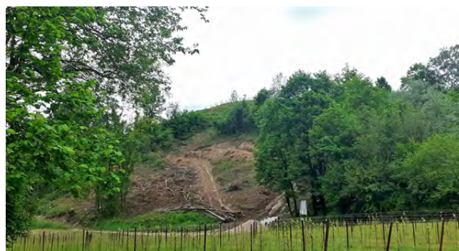
Fig. 3: Earth excavations and deforestation in the Tarzo hills for new vineyards, 8 May 2024.
