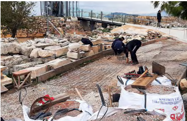
Fig. 5: A pathway out of the boundaries of the tourists' routes on the Acropolis in the process of being paved with reinforced concrete. Above left, the new elevator. Above right, behind the tree the Erechtheion. View from southwest (January 2023)
