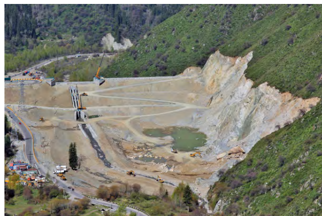
Fig. 3: Mudflow protection dam, Big Almaty Canyon, former territory of Ile-Alatau National Park (May 9, 2023).
