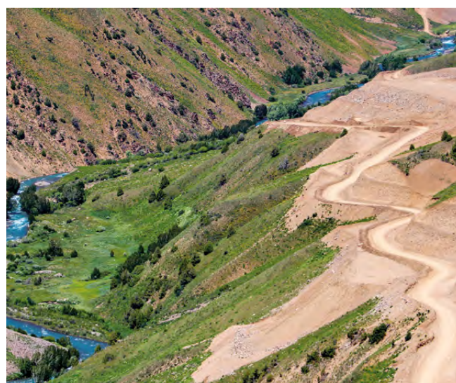
Fig. 1: The new road to the Chaarat mine apparently passes through the Sandalash site of the World Heritage property, where the protected area status has been abolished. Photo: www.chaarat.kg
