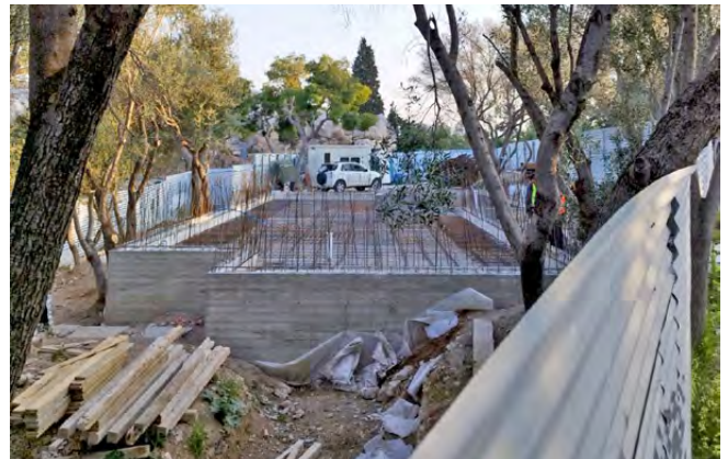
Fig. 6: The foundations of the new ticket office buildings, with vertical rods for the reinforcement of the walls. At the background the rock of the Areopagus. View from the south. (2024)
