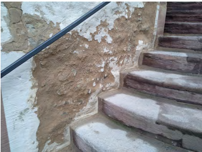
Fig. 4: The outside wall of the City Hall exhibits serious humidity after a 12-year restoration which had cost 14.4m EUR. Photo: Henning Frase
