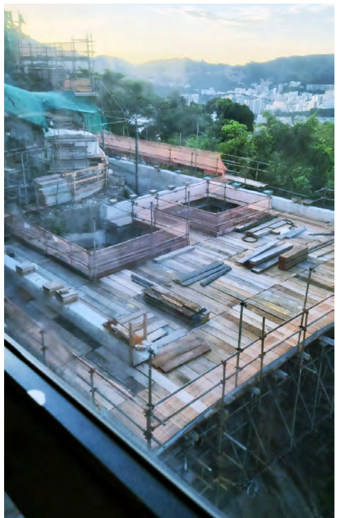
Fig. 16: Despite its low quality, this is a rare image of the platform being built before the judicial embargo and its subsequent concealment by large green canvas covers. Is such an expansion acceptable? Photo: Movimento Pão de Açúcar sem Tirolesa
