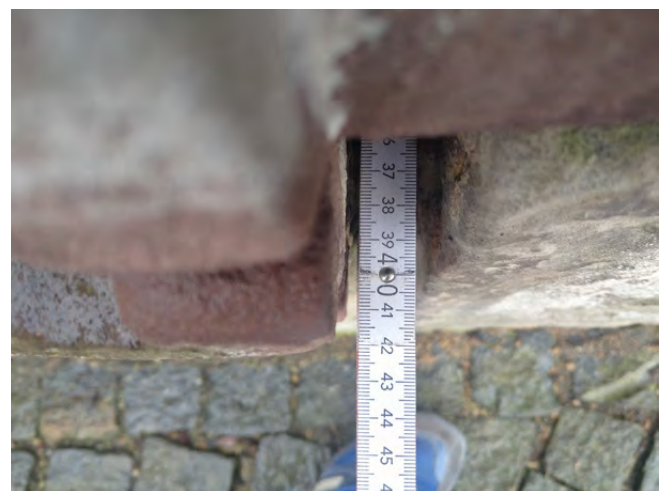
Fig. 7: Open joints in the exterior staircases of the Imperial Palatinate are up to 40cm deep. Photo: Henning Frase
