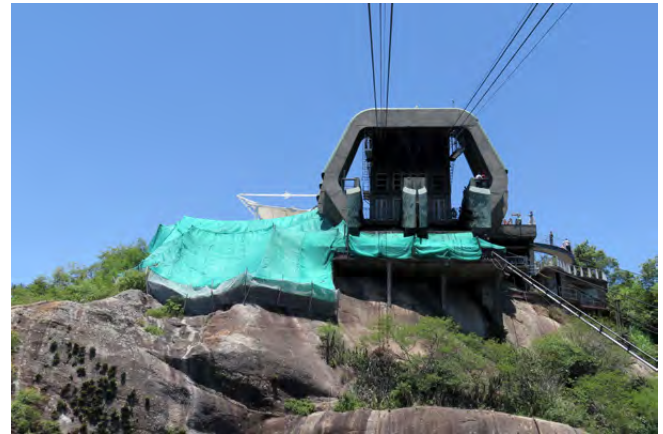
Fig. 6: After the judicial embargo, the company covered everything with thick green canvas to hide from visitors the extent of the damage already done. Photo: André Ilha
