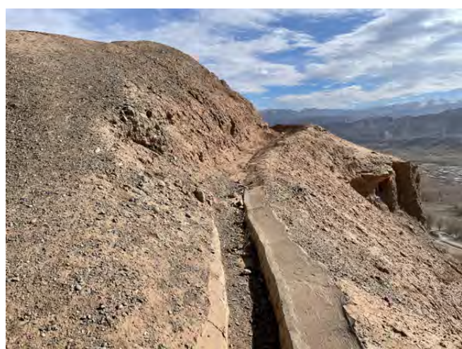
Fig. 8, 9: The drainage system above the Buddha niches which need to be maintained.
