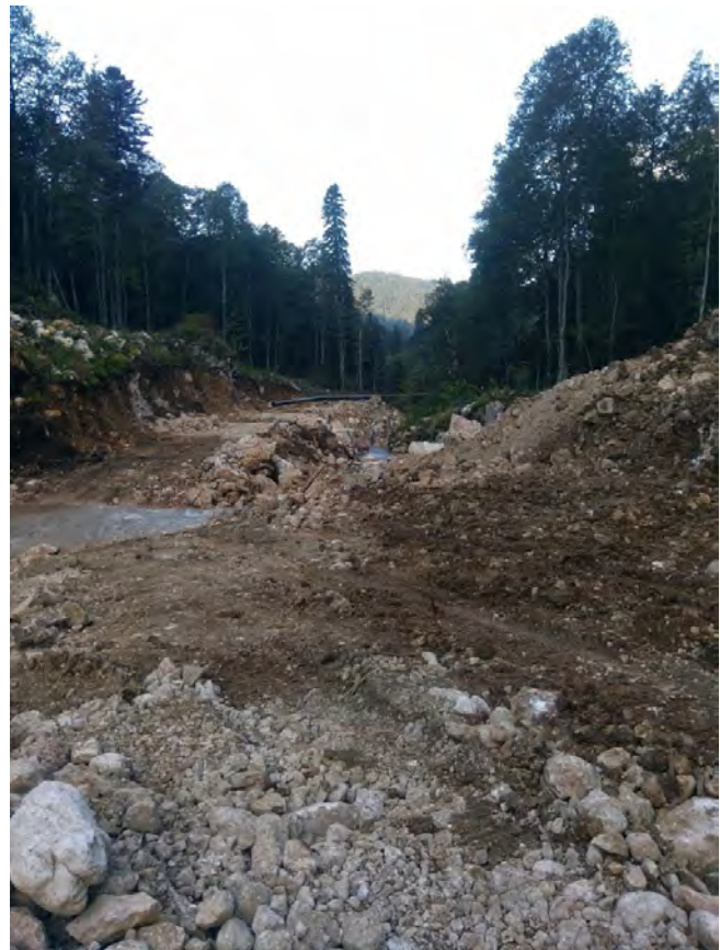
Fig. 6: Destruction caused by the construction of a water pipeline. Photo: The authors
