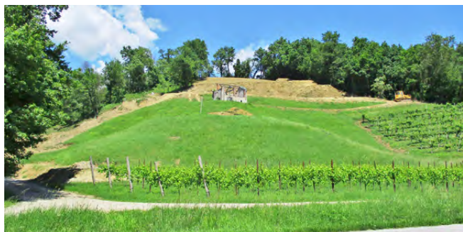
Fig. 2: Earth excavations and deforestation of the Campea hill for new vineyards, 30 May 2021.
