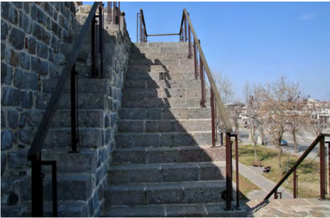
Fig. 5: Ugly railing appearance on the city walls. Photo: Pinar Can, DKVD Diyarbakır City Archive, 5.03.2025
