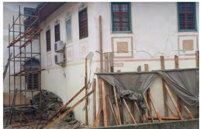
Fig. 4: Russia’s so-called ‘restoration’ of the Khan’s Palace and the potentially irreparable damage it has caused.
