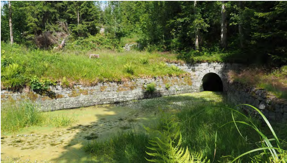
Fig. 7: The Lautenthaler Kunstgraben includes a number of technical features such as stabilizing walls, tunnels, channels, weirs, ponds and scoop wheels which diverted water to the various mines in the Harz. Its dilapidated state has been criticized by NGOs. Photo: Anja Deubl / NDR
