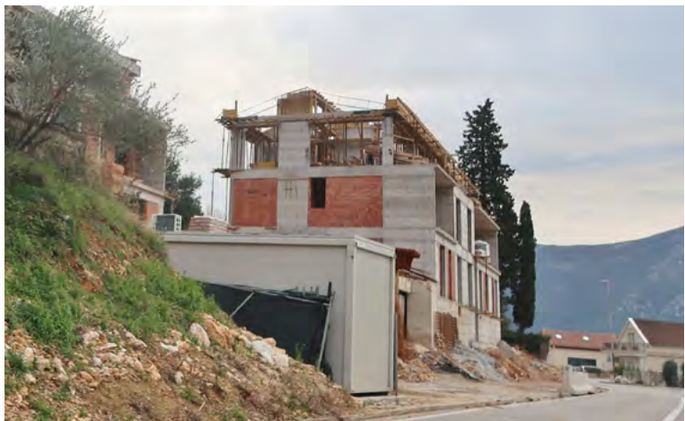
Fig. 8: Example of structures currently under construction in Ljuta under the provisions of the Spatial Urban Plan for Kotor Municipality (SUP). Although the basement should be an underground part of the structure, this is often not the case. As a result, buildings presented in the plan as having just first floor and attic usually comprise four full levels, with large volumes that deviate from traditional structures, and disrupting the historic urban fabric. The largest traditional buildings, palaces, typically feature a ground floor, two floors, and an attic with a belvedere. But those new structures vastly exceed the traditional structures, including even the palaces.
