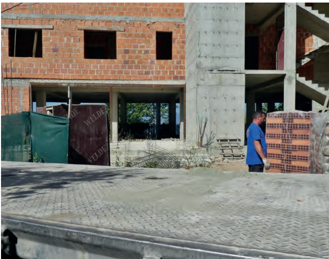
Fig. 2: Illegal construction continues at a lakeshore hotel on 3 July 2019, the same day as the Macedonian delegation addresses the World Heritage Committee.
