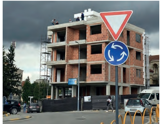
Fig. 3: Although a construction moratorium has been announced in the Ohrid region on 8 August 2019, it does not cover work at the numerous buildings that are already under construction, here on 26 September 2019. Photo: Ohrid SOS
