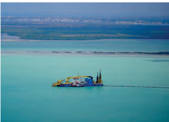
Fig. 3: Dredger operating in proximity to Lamu Old Town for the construction of the first of 32 berths for Lamu Port, with significant turbidity in Manda Bay, April 2019. Photo: Save Lamu
