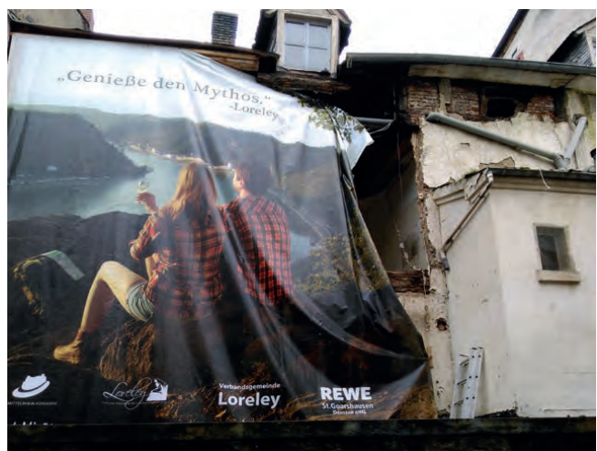
Fig. 7: Houses decay. Their repair is not economical.
