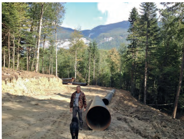
Fig. 1: Construction of the water intake and water supply main to the settlements of Maikop district and the city of Maikop (first start-up facility). Photo: Yuri Vorovsky
