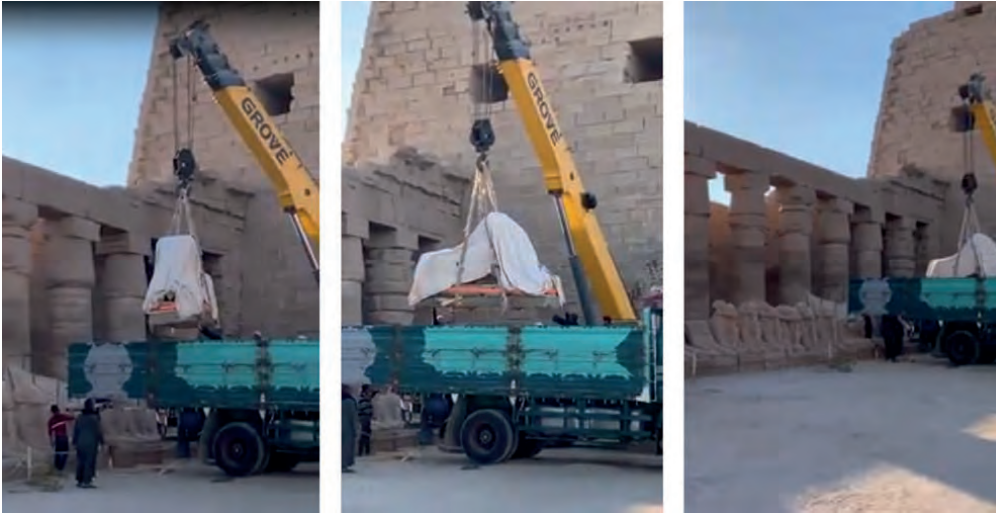
Fig. 4: Circulated photos of the relocation procedure of ram-headed sphinxes from Karnak on 8 January 2020. Source: www.facebook.com
