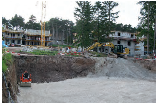
Fig. 9: GESIBA residential buildings (6) and (8) under construction; the construction pit for residential building (7) in the foreground. Photo: Christian Schubböck
